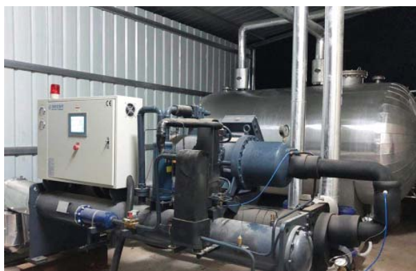
Chemical Factory, Low-temp Water-cooled Chiller
