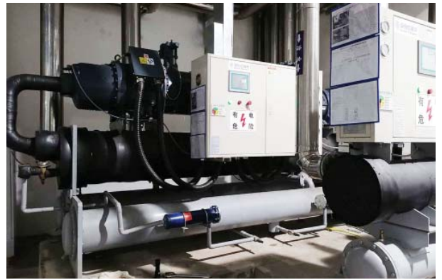
Electroplating Factory, Low-temp Water-cooled Chiller
