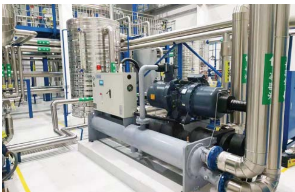
Dairy Factory, Low-temp Water-cooled Chiller
