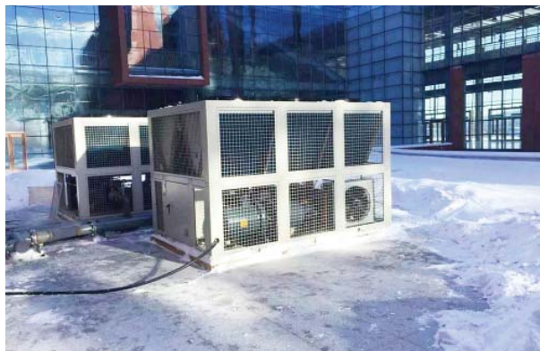
Stadium, Stationary Air-cooled Chiller
