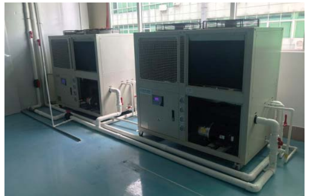
PCB Factory, Portable Air-cooled Chiller
