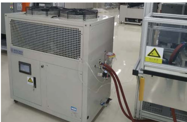
Laboratory, Air-cooled Chiller
