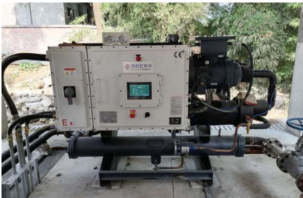
Plastic Industry, Explosion-proof Chiller
