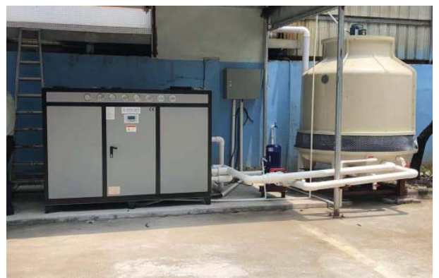
Silicone Strip Factory, Portable Water-cooled Chiller
