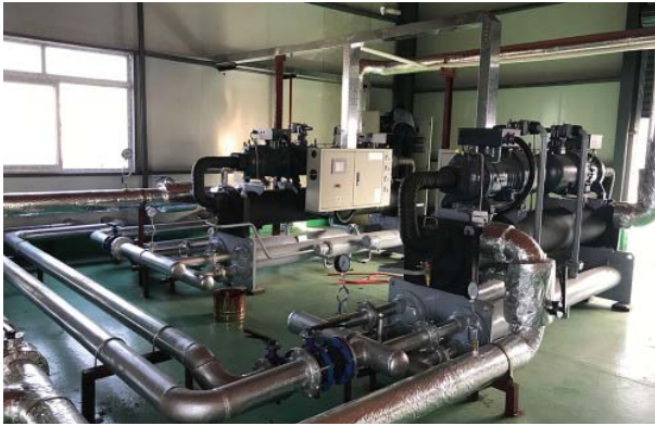
Sanitary Ware Factory, Water-cooled Chiller
