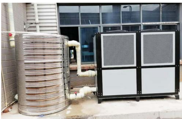
Printing Factory, Air-cooled Chiller
